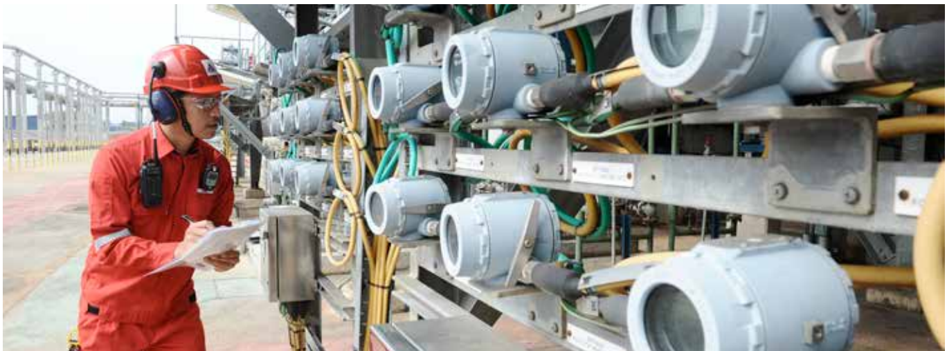
Routine operational inspections are conducted regularly to ensure all systems are working with optimum efficiency.
