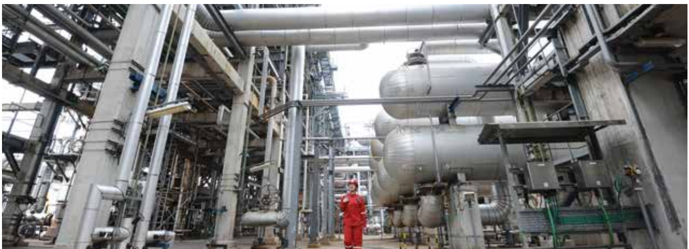
Rigorous preventive maintenance, inspection and process safety programmes have been in place for over a decade to uphold the integrity of the refinery.
